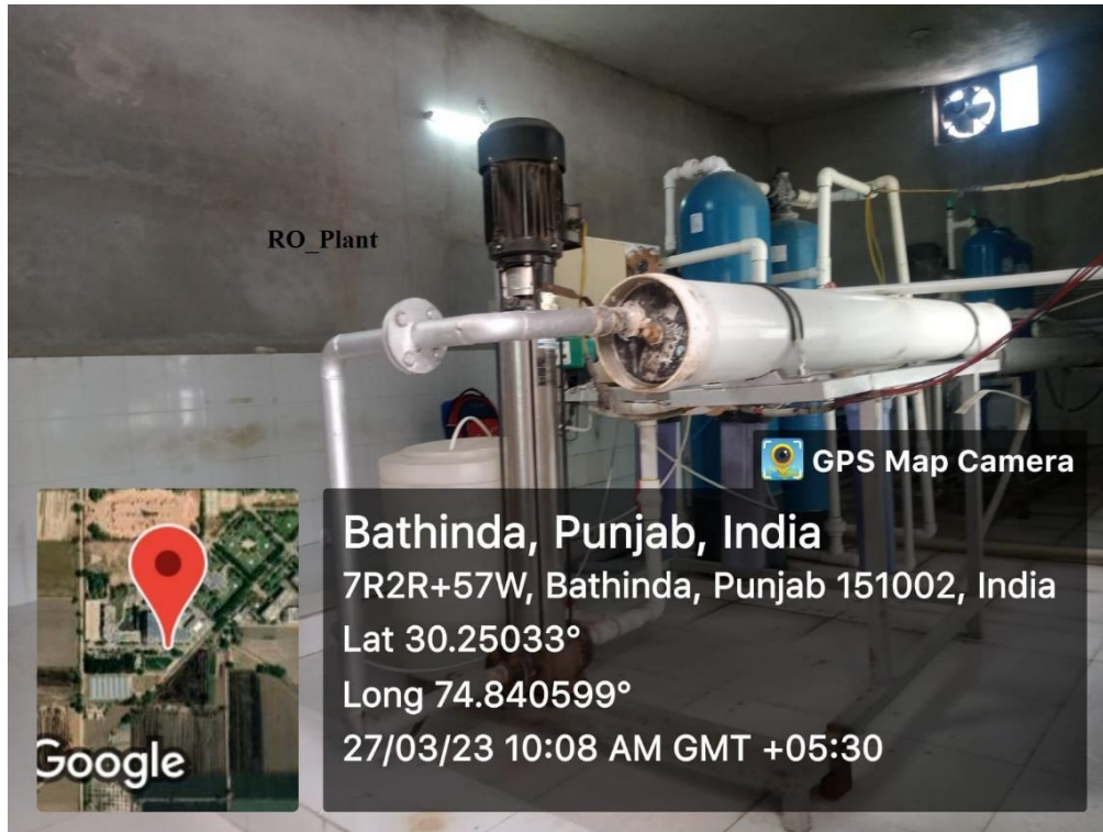
Figure 1: Water conservation (RO Plant)
