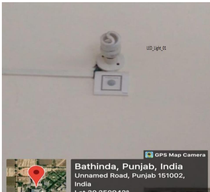
Figure 12: Alternate sources of energy and energy conservation measures (Power efficient equipment)
