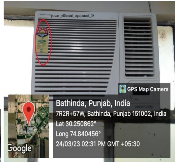
Figure 6: Alternate sources of energy and energy conservation measures (Power efficient equipment)
