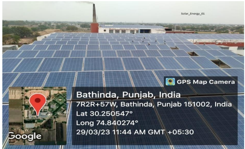
Figure 1: Alternate sources of energy and energy conservation measures (Solar Panels)
