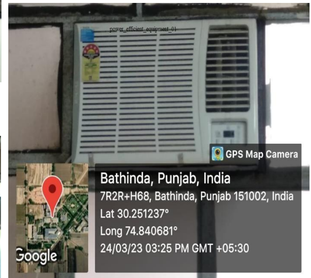
Figure 8: Alternate sources of energy and energy conservation measures (Power efficient equipment)
