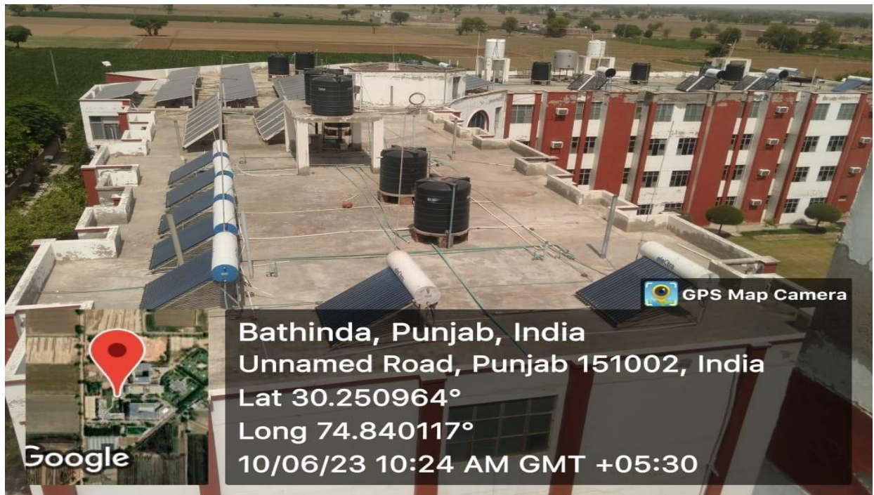
Figure 4: Alternate sources of energy and energy conservation measures Solar Geyser
