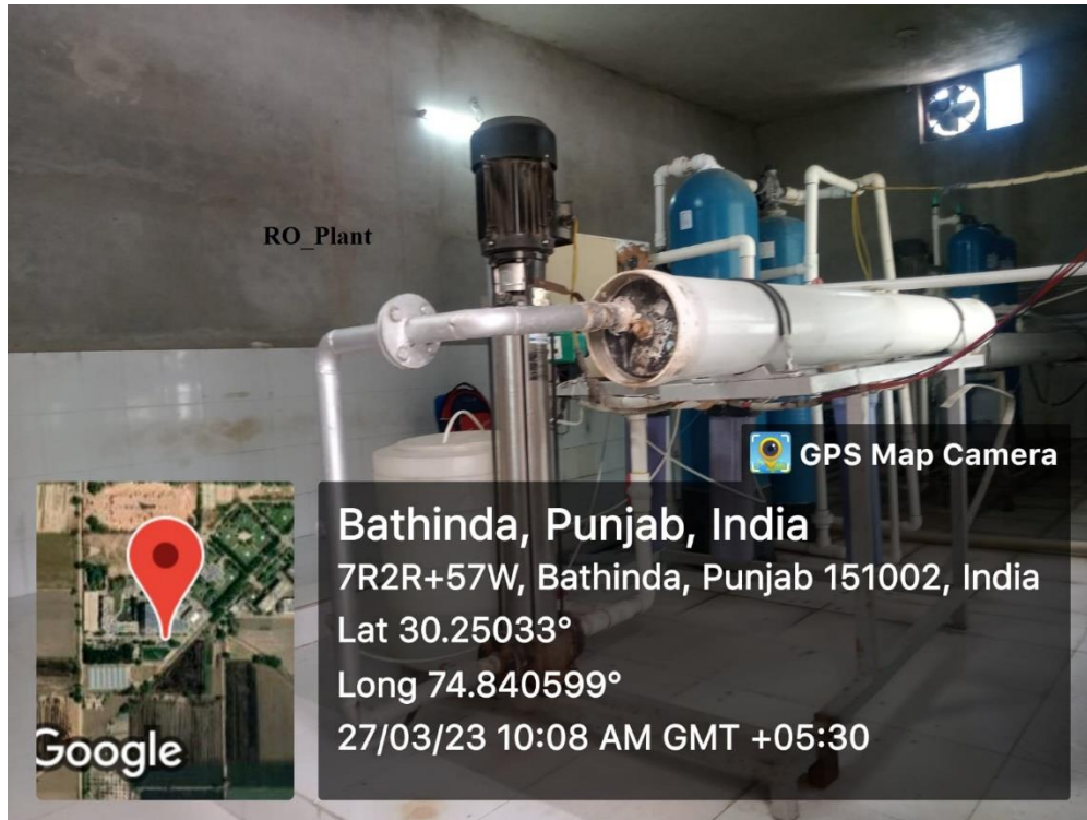
Figure 1: Water conservation (RO Plant)
