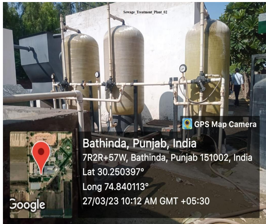
Figure 3: Water conservation (STP Plant)
